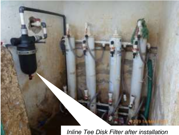
Inline Tee Disk Filter after installation
