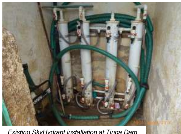
Existing SkyHydrant installation at Tinga Dam
