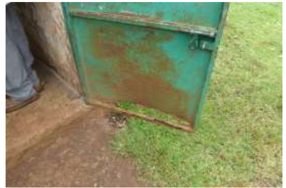
This is the only area of corrosion identified at all kiosks
