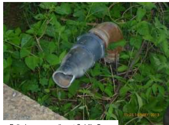
Failed pump coupling at Ochillo Dam
